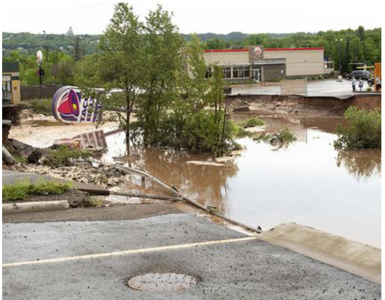
A Taco Bell drive-through caved in and washed away after heavy rains and flooding in Houghton, Mich. on June 17, 2018 | David Archambeau, AP
