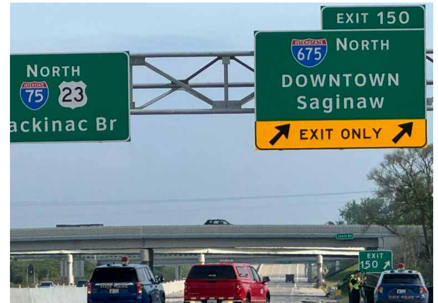
MOTORISTS TRAVELING ON I-75 IN SAGINAW COUNTY SHOULD PREPARE FOR TEMPORARY CLOSURES AND ROLLING SLOWDOWNS AS MDOT CONDUCTS UTILITY WORK NEAR CRANE ROAD.
