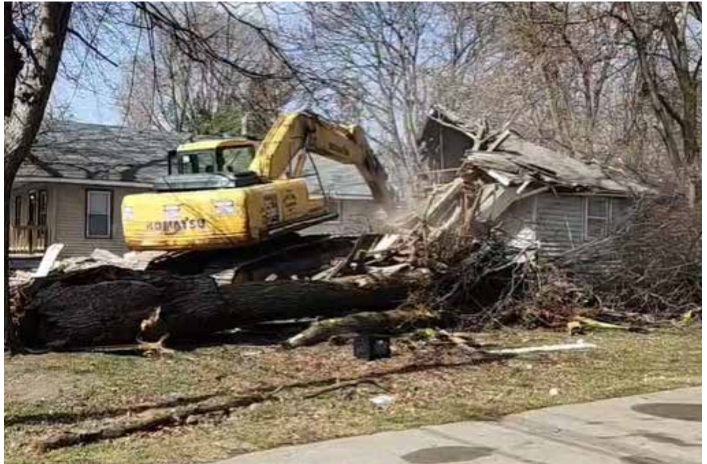
DEMOLITION UNDERWAY AT 1808 W. GENESEE AFTER A LARGE TREE COLLAPSED ONTO THE HOME ON SATURDAY, MARCH 14.
